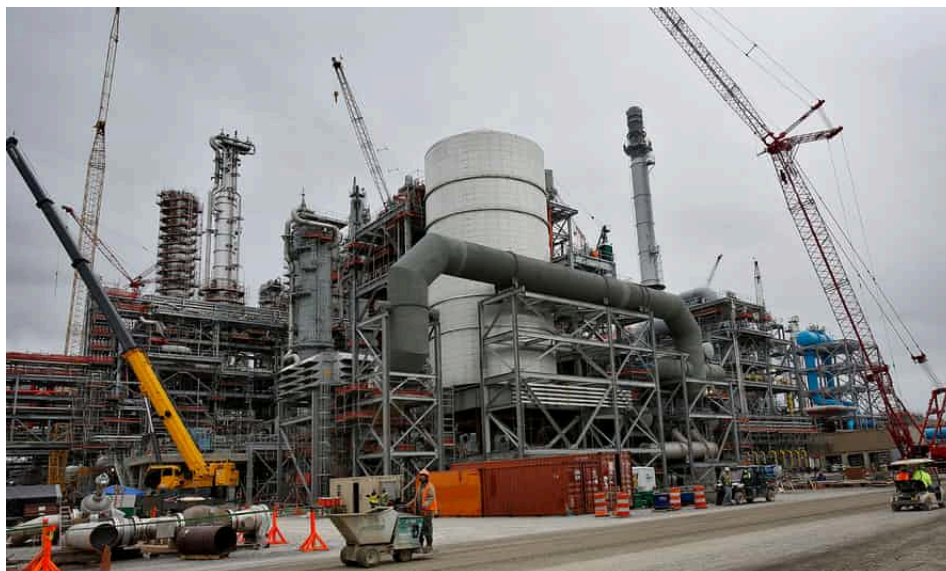
Cranes stand at the construction site for Southern Co's Kemper County power plant on 25 February 2014. Photograph: Bloomberg/Bloomberg via Getty Images
