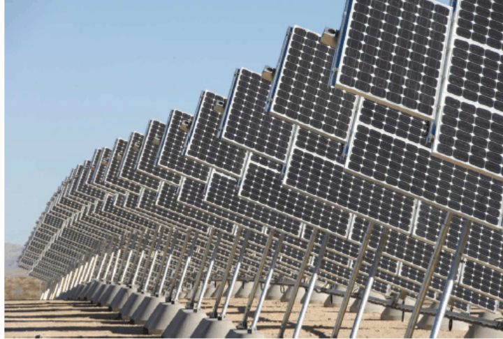
Figure 30. Nellis AFB Photovoltaic Array Detail
