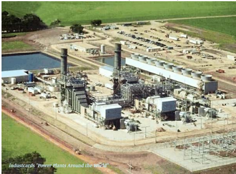
Figure 16. Representative Combined Cycle: McClain Plant (Oklahoma)
